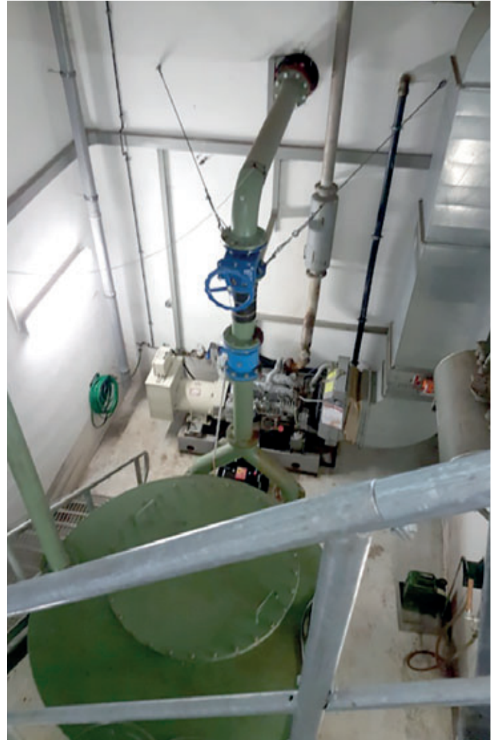
Blick in das Pumpwerk
